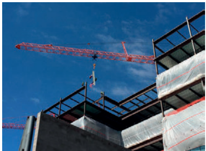
The structural topping out for Union Tower West took place on April 9, 2015 with both the state of Colorado flag and the U.S. flag proudly displayed.
