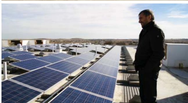
A delegate inspects the 98kW rooftop solar array at Josephine Commons.
