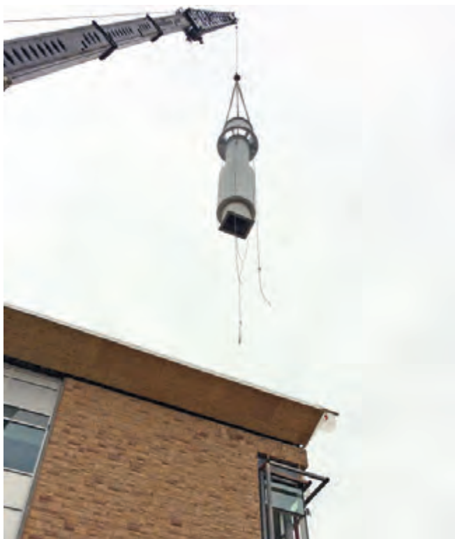
Exhaust stack being hoisted to roof of Enzi Building. Photo by Kuck Mechanical.
